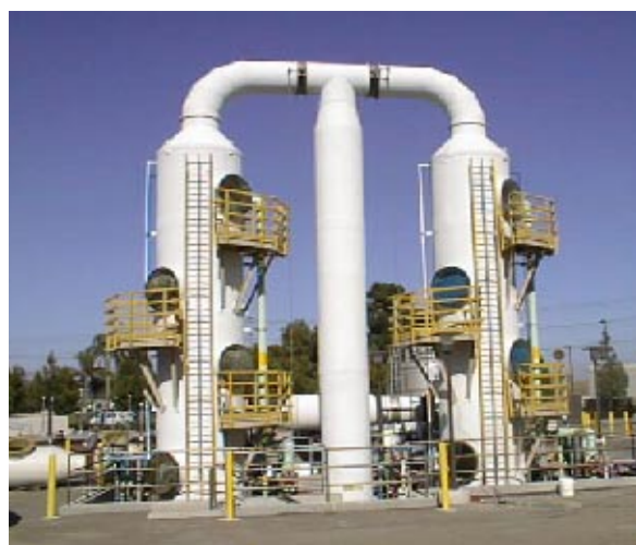
Chemical scrubber in Orange County wastewater treatment plant converted to a biological scrubber.
