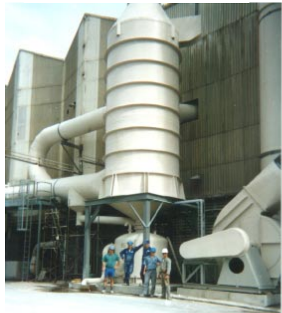
Wet cyclone scrubber at fertiliser works.
