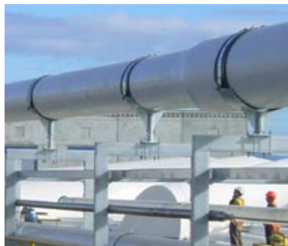
FRP duct and supports at a wastewater treatment plant.
