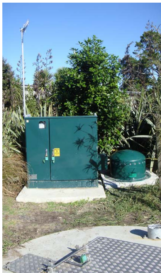
Mangawhai Village Green Dome Odour Filter alongside the pump station and control cabinet. The duct and part of the Green Dome are buried to minimise visual impact.
