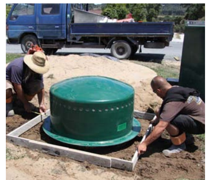
Backfill base module and prepare to pour concrete pad for top module bolting.
