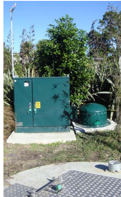
Green Dome Odour Filters for pump stations and air relief valves ... low profile and green for minimum visual impact.
