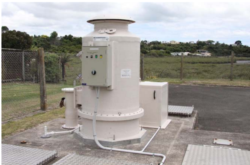
Photo 4: Otumanga Pump Station: Carbon adsorption bed with inlet filter, fan & acoustic housing
