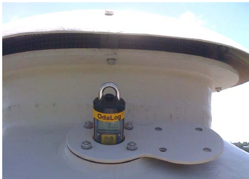
Photo 1: OdaLog Gas Data Logger on Carbon Bed Outlet
