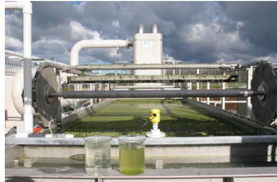
Flotation tank where algae, phosphorus and suspended solids are removed from the oxidation pond effluent. The treated water is clear (left hand container).
