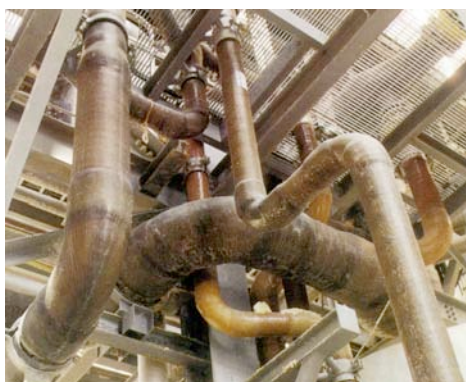
Fig 1: FRP pipes at Kinleith Pulp & Paper Mill
