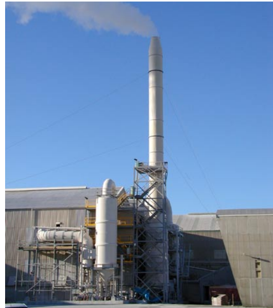
BAN Awarua fertiliser plant fluoride scrubbing system
