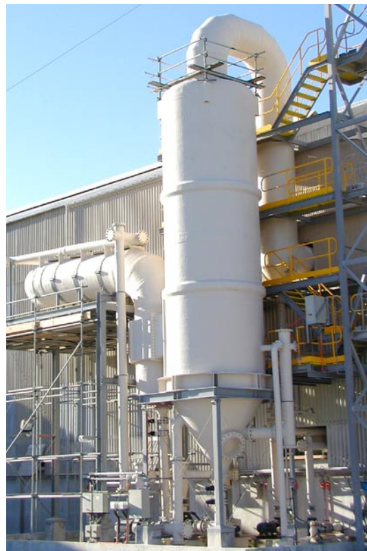
High efficiency void tower in fluoride scrubbing train
