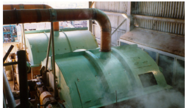
Fibreglass cover over pulp washers for chlorine containing fumes. Covers are able to be lifted clear by overhead gantry when access is required to washers for maintenance.
