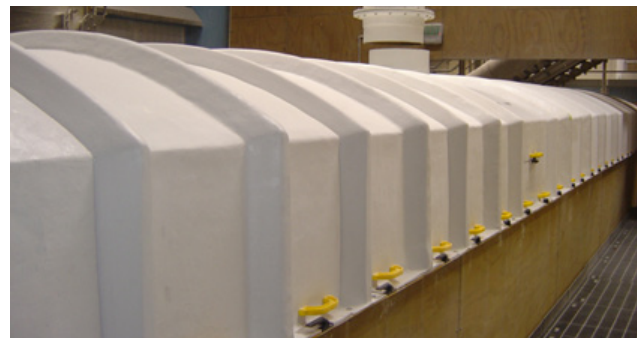
Segmented fibreglass cover over conveyor at biosolids plant at municipal wastewater treatment plant.
