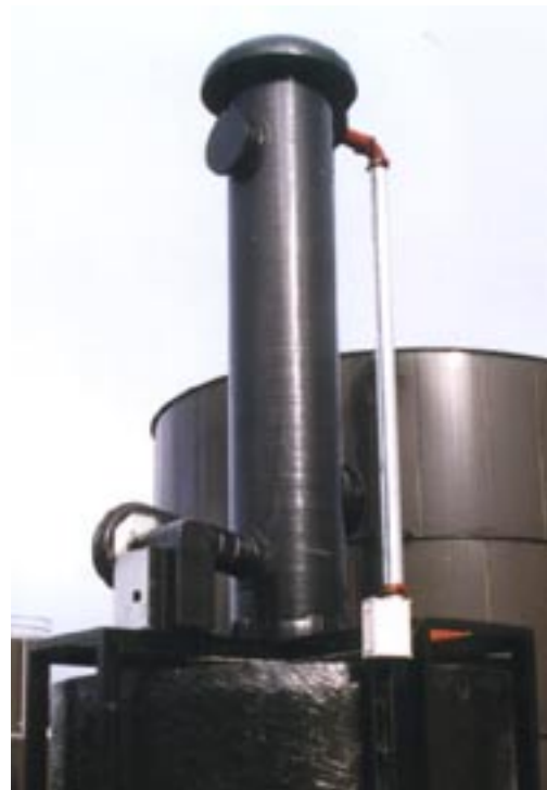
Degasser for removing carbon dioxide from water mounted on top of a concrete storage tank.
